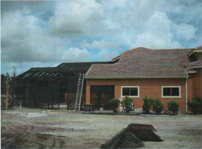
LEFT SIDE VIEW (AIR CONDITIONER SLABS) 04-07-2008
