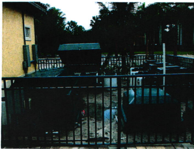
Pool Equipment 12 July 2013
